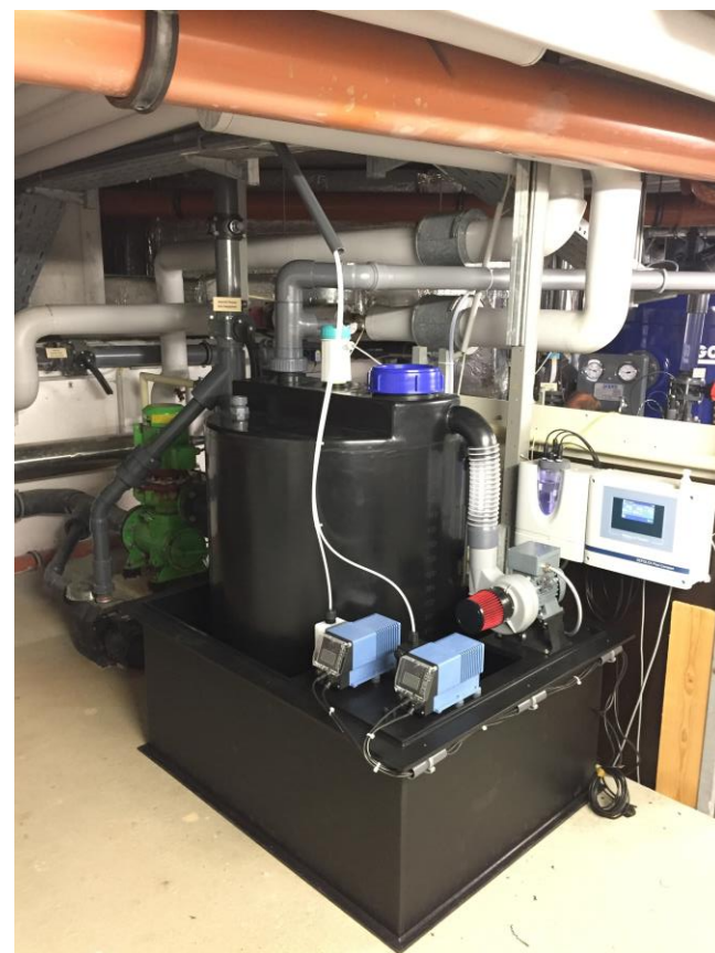
Hypochlorite storage and dosing
